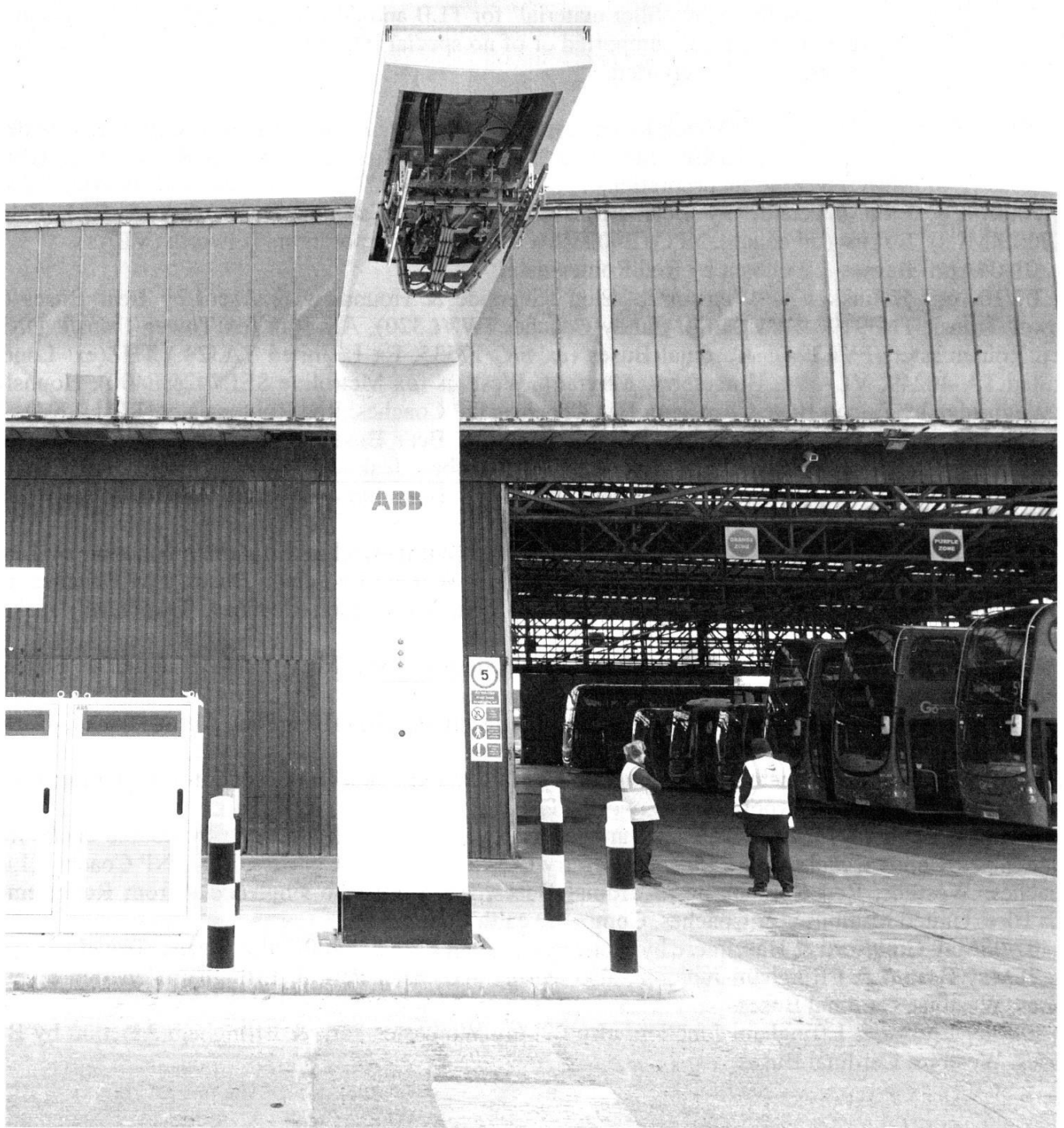
Bexleyheath Garage – Pantograph installed but power supply is still “Coming Soon”.
